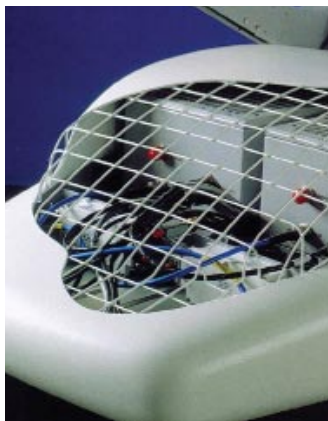
Two HPAs located within the antenna assembly
